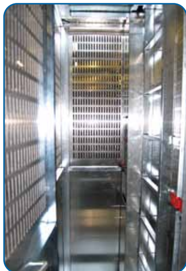
Interior de cabina Interior of the cabin
